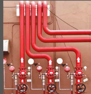
ULTRA MODERN FIRE FIGHTING SYSTEM
